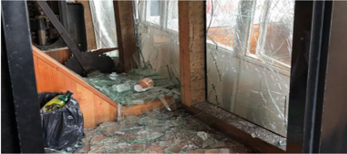
Figure 11. Damage Caused by the Accident
