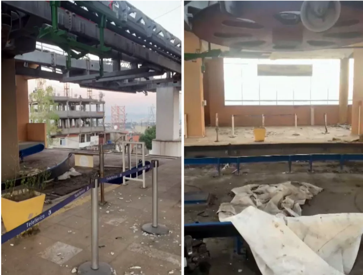
Figure 13. Deteriorated Cable Car Structure in Complexo do Alemão
